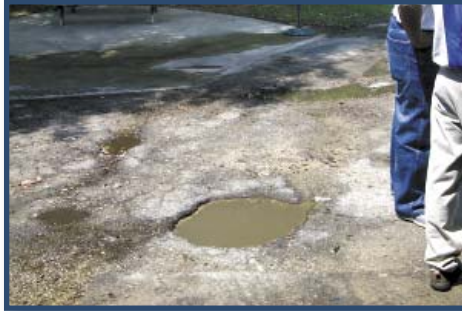
Figure 14. Dirty water in this puddle just outside the car wash tunnel indicates some car washing took place outside the wash tunnel, allowing dirty water to run onto the ground instead of into the collection pit.
