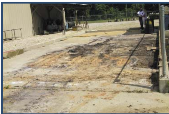
Figure 16. The rain falling onto this wash pad can be diverted to the stormwater sewer via a removable rain water dam. This prevents the recycle system from overflowing due to excess volume. The wash pad must be thoroughly cleaned before diverting the rainfall off the pad and into the storm sewer.
