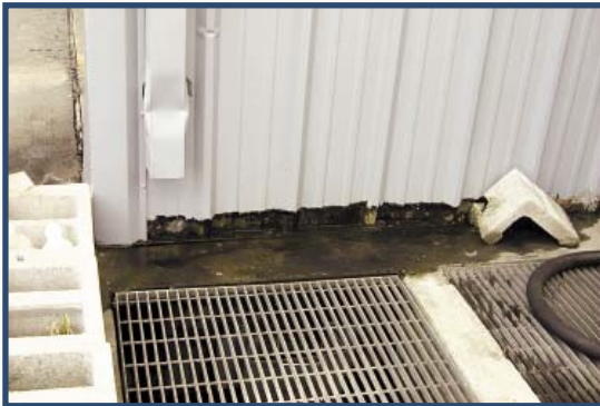
Figure 15. The collection pit at this car wash facility is located outside, adjacent to the wash tunnel. The pit is not covered, there is no overhang, and the downspout brings rain water right into the pit. This situation must be corrected.
