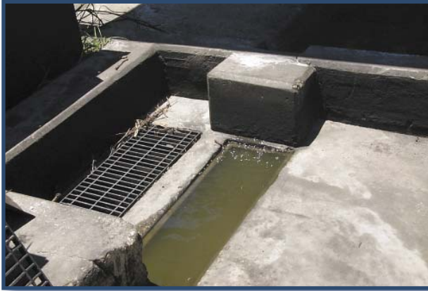
Figure 18. The wash pad at this facility is equipped with a stormwater diversion valve.
